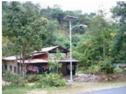
Compound / Housing Estate Lighting
